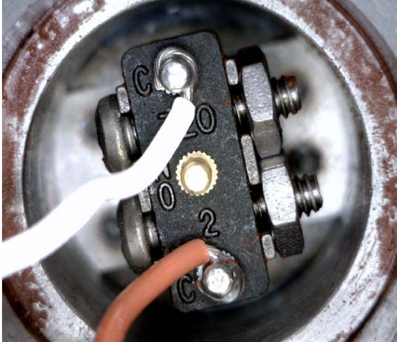
Electrical Assembly - Functional; good condition
